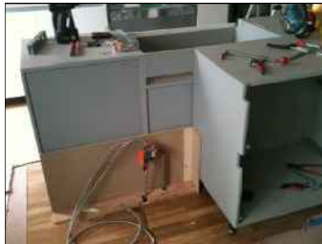
EXAMPLE - ELECTRICAL CONDUIT AT ISLAND
