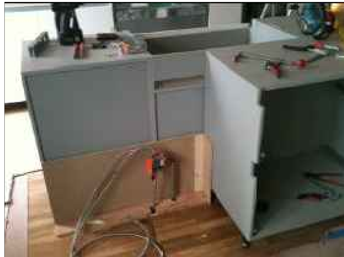
EXAMPLE - ELECTRICAL CONDUIT AT ISLAND
